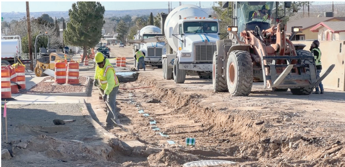
Crews install a new 18-inch wastewater line along Graphite Drive, Mace Street and Conley Road.
